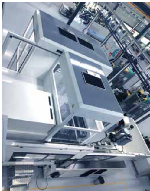
Overview of the installation, showing an Engel injection moulding machine fitted with two canopies, a fixed one at the back with two filters, and the sliding canopy at the front with one filter unit.
